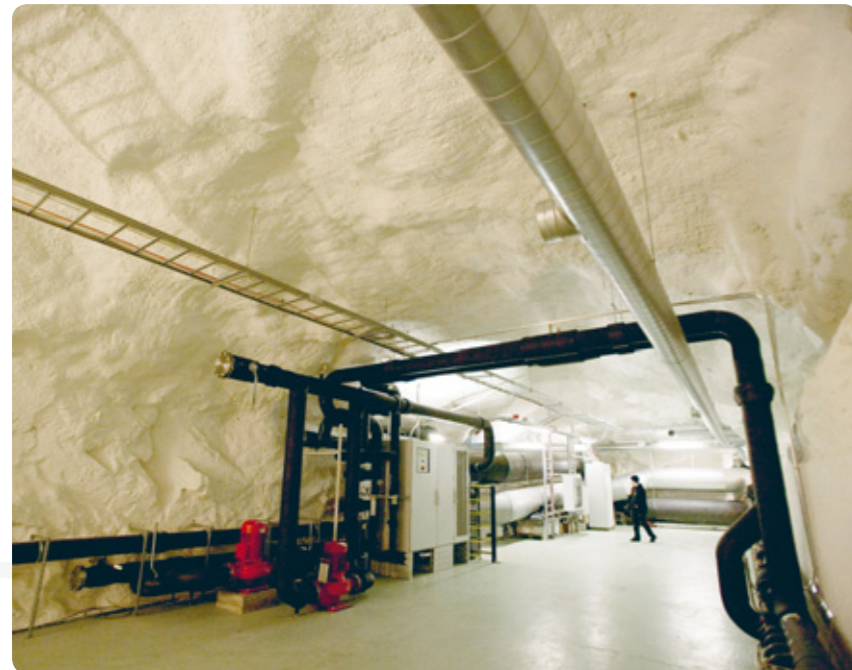
District cooling equipment in the Uspenski data centre, which was inaugurated in October.
